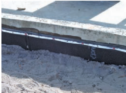
Extra measures were taken to ensure the foundation and shallow basement were waterproof.
