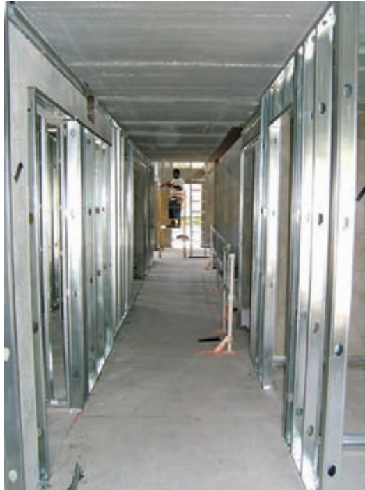
Steel framing was used for faster installation into concrete exterior, floors, and ceilings.
