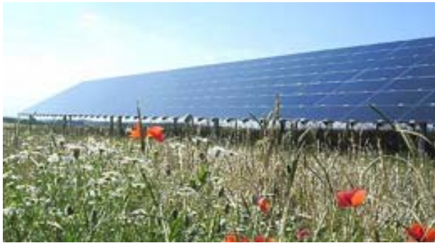
Figure 1: Thin-film CdTe 1,400-kW thin-film solar installation.
