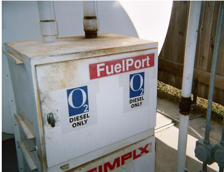
Figure 12. Outside of O 2 Diesel fuel port on storage tank at JCT
