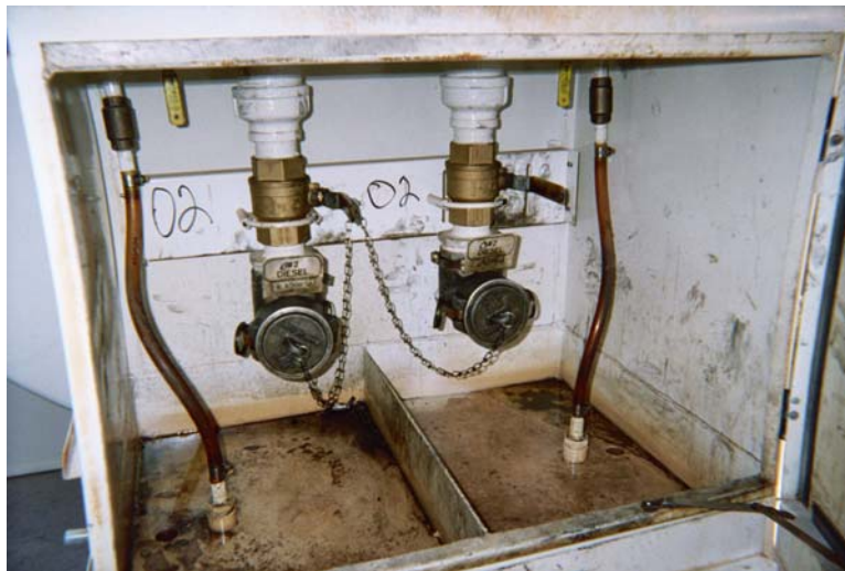
Figure 13. Inside of O 2 Diesel fuel port on storage tank at JCT
