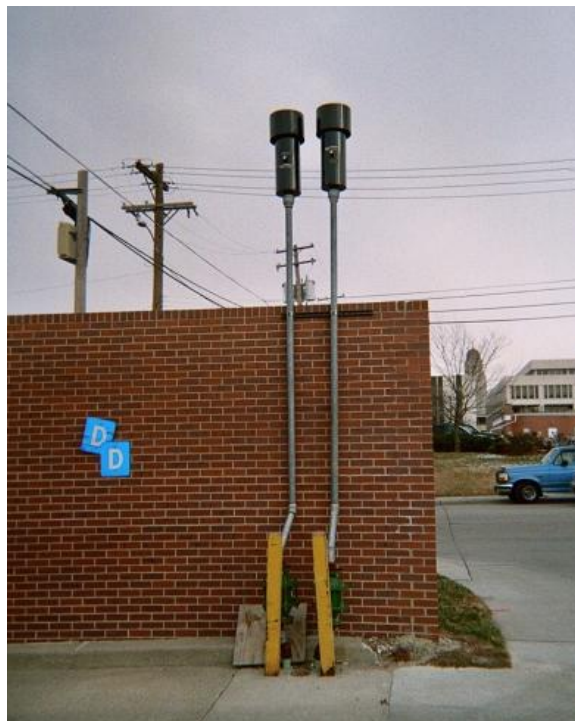
Figure 15. Flame arrestors and desiccant filters on underground storage tanks at Lincoln StarTran
