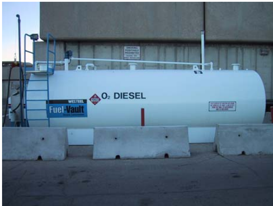
Figure 2: TYPICAL O 2 DIESEL™ ABOVE-GROUND STORAGE TANK EQUIPPED WITH FLAME ARRESTORS, DESICCANT FILTERS, AND PROPER PLACARDS.
