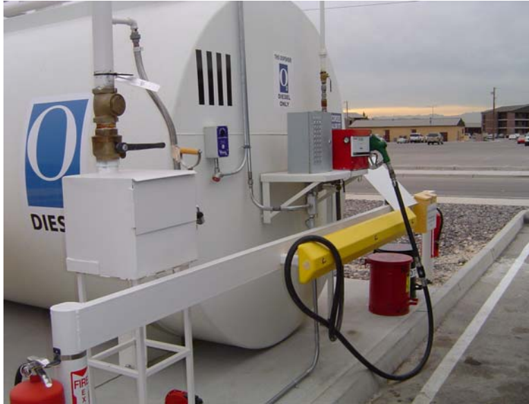
Figure 2. O 2 Diesel fueling station at Nellis AFB
