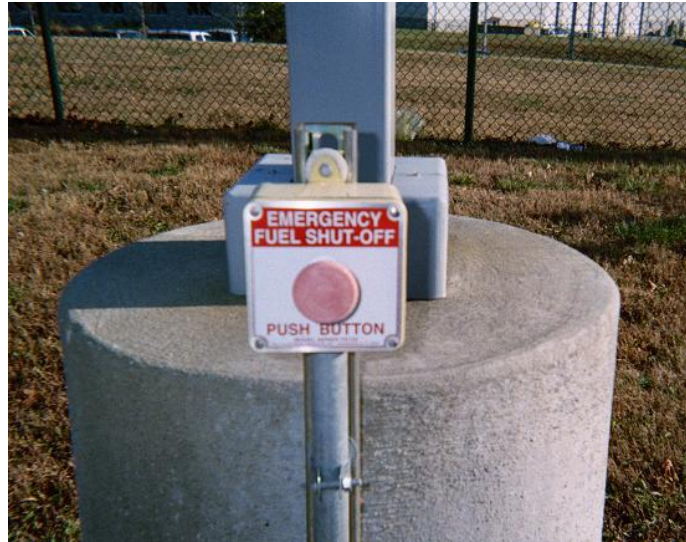
Figure 10. Emergency fuel shut-off button at JCT
