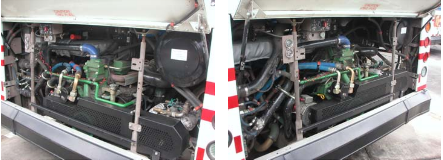
Photos 3-3 and 3-4. Views of John Deere 8.1 L engine installed in New Flyer Bus
