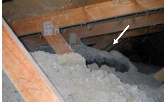
Figure 11. Ductwork partially buried in attic
