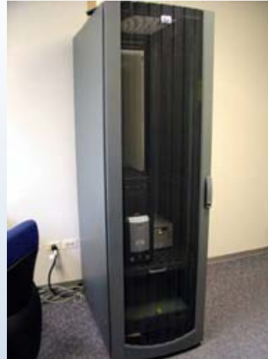
Server, workstation, tape backup and UPS
