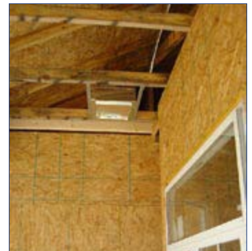
Air Intake being installed in a porch overhang to provide fresh air to attic HVAC.
