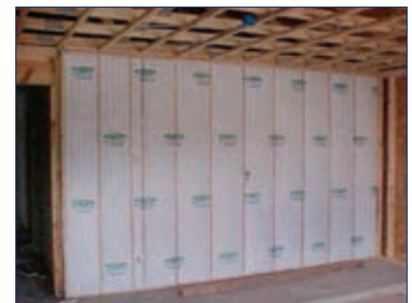
Artistic Homes uses advanced features recommended by Building America including 2-by-6-framing, allowing for R-23 blown-in insulation in the walls and R-38 in the ceiling, application of wrap and sealing to create a continuous air barrier from slab to ceiling, sealed ducts with mechanical ventilation, and transfer grilles between room for even air distribution and less drafts.
