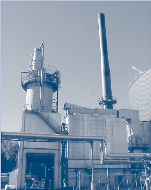
Power plant boilers at the Solutia site
