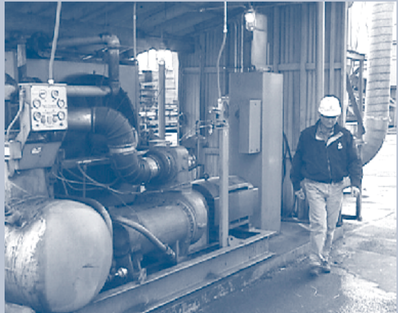
The largest of three rotary screw compressors at the mill is this 300-hp unit.
