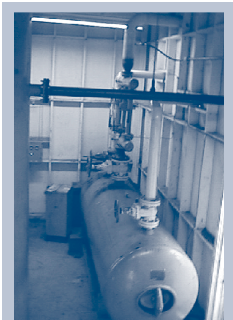
To stabilize system pressure, compressed air is stored in containers such as this 800-gallon horizontal unit.
