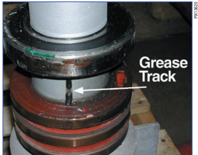
Figure 3. Lower yaw bearing and slirings. Note grease track from yaw bearing to top slirings track.
