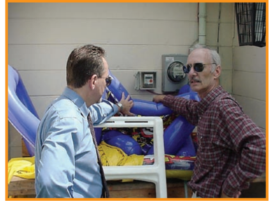
After moving aside pool toys, Jeff Curry explains operation of the utility's meters for domestic hot water on the home of Maureen Roe. Ms. Roe was the first customer to receive a solar hot-water installation from the Lakeland Electric Company.
