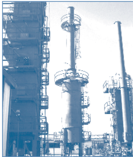
Test furnaces for high-efficiency, ultra-low-emissions, integrated process heater systems. PIX 11012
