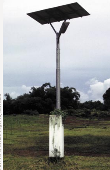
A PV module in a rural area in China.
