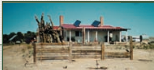
Pueblo of Laguna solar electric installation
