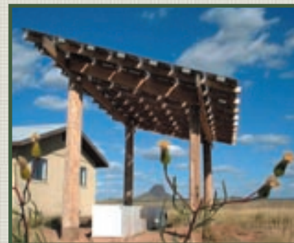
Solar electric array on Navajo home
