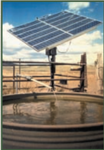
Ute Mountain Indian Reservation PV water pumping
