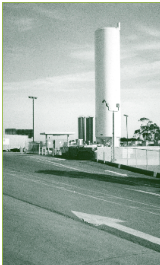
Figure 3. LNG Fueling Station at SF Recycling & Disposal
