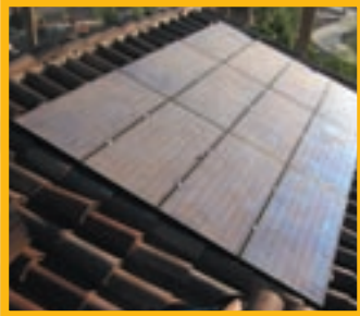
Solar electric panels mounted unobtrusively on the roof on the back side of the house.
