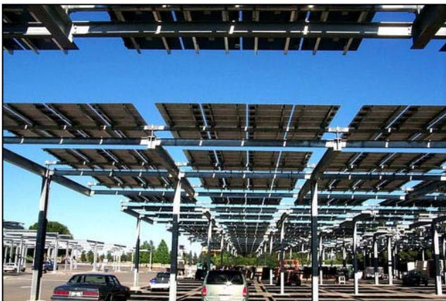
Grid-connected PV parking lot system
