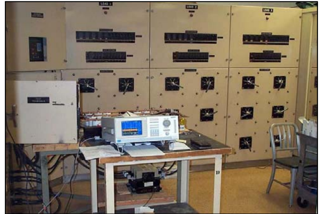
Three-phase anti-islanding test equipment at UL
