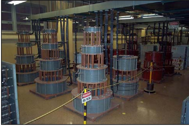
Inductive load banks UL uses for anti-islanding tests at its Northbrook, Illinois, facility
