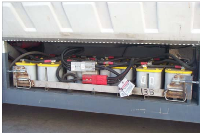
Lead acid battery pack in a hybrid bus.
