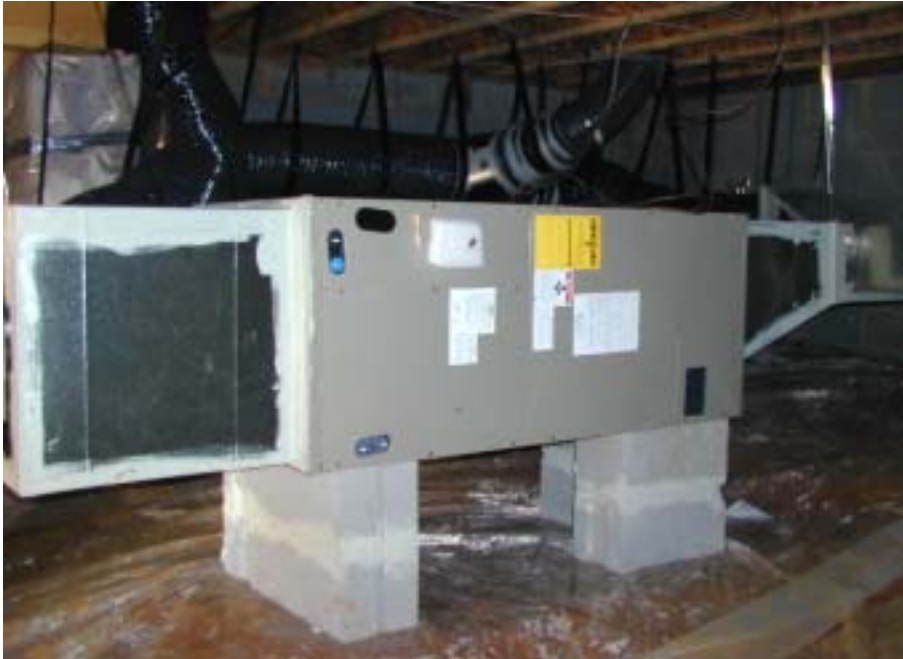
Figure 7. Locating mechanical equipment responsible for air movement in a conditioned space, such as this conditioned crawlspace, means that it is not subject to the cold and extreme hot and humid circumstances that it would experience if it was located in an attic, vented crawlspace, or the outdoors.
