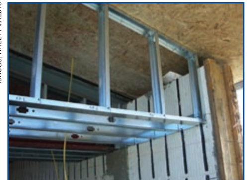
Insulated concrete forms, steel beams, and structural insulated panels make up the building enclosure.
