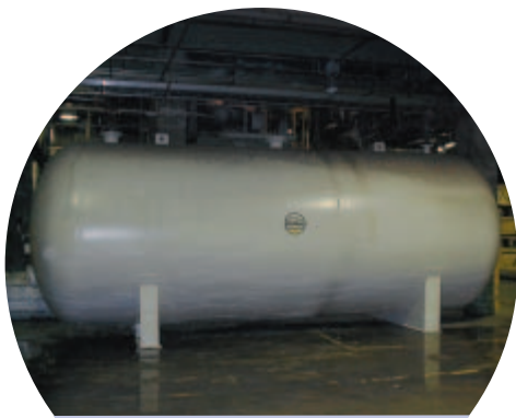
New 10,000-gallon compressed air storage tank
