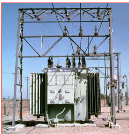
When local electrical subsystems fail, the cost to business can be substantial.
