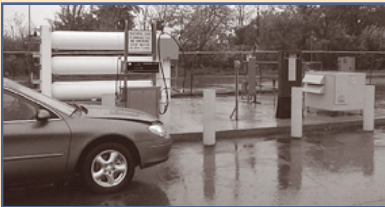
New York built 30 CNG stations with an eye on future expansion.
