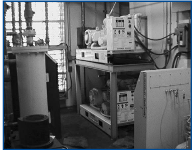
Printing machine redesign and measures to reduce end-use requirements allowed Harland Publishing to achieve greater efficiency through reduced compressed air demand.
