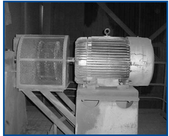
New mechanical ASD installed on the baghouse fan system.
