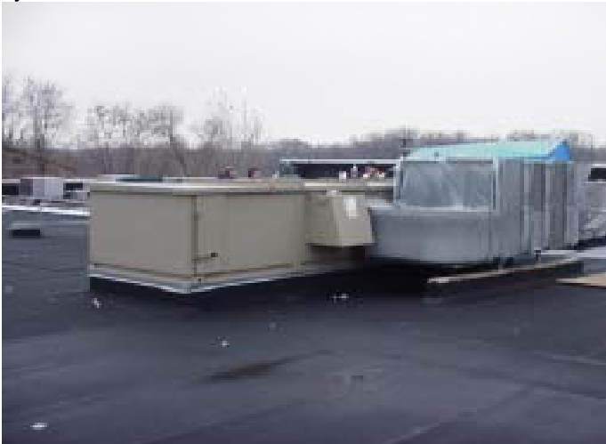
Packaged CHP system incorporating desiccant dehumidification system
