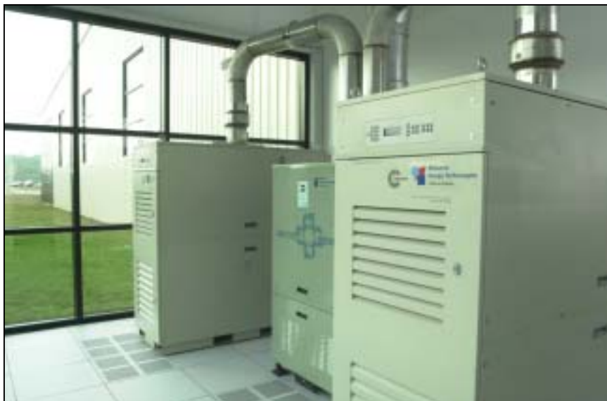
Two-turbine CHP installation
