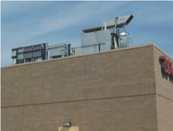
Packaged CHP system that includes a 30-kW microturbine, heat recovery system, and desiccant dehumidification system
