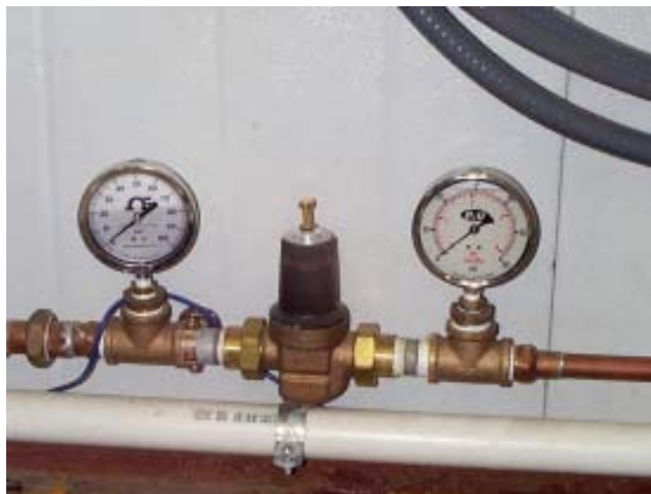
Figure 5. Inlet pressure monitoring and regulation system
