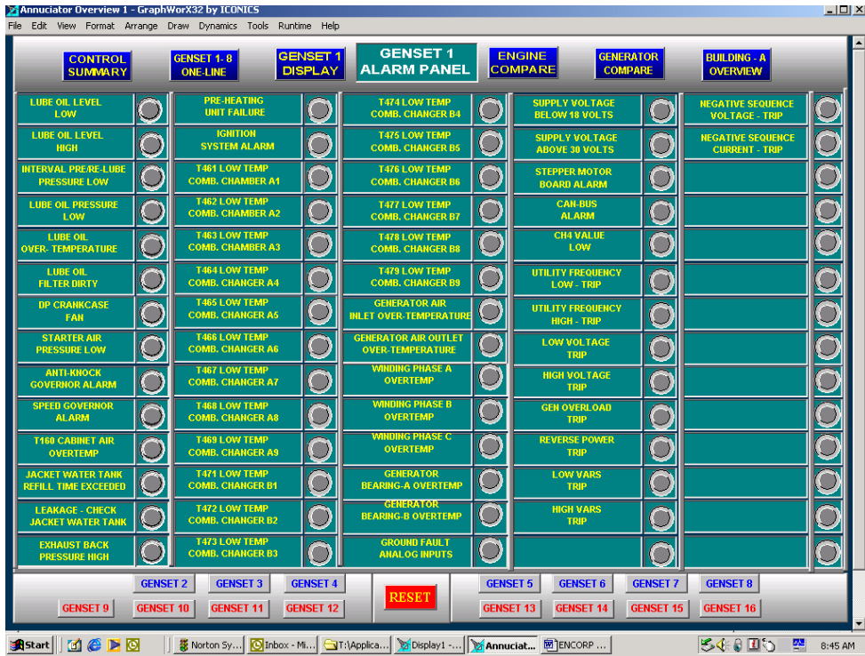
Figure 8: Generator annunciator display
