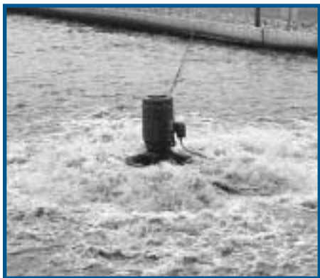
Ellensburg's dilemma: replace or rewind a 50 hp aerator motor?
