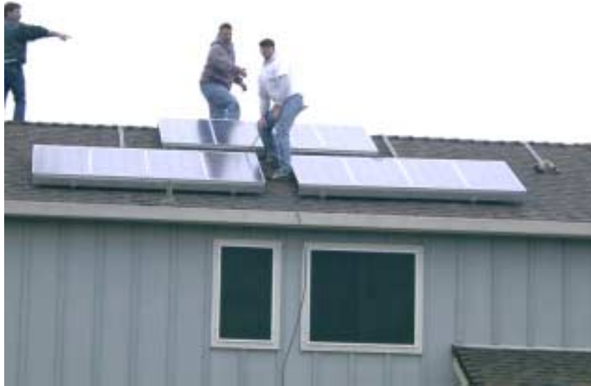
Figure 11. Final Design with Three PV Panels in Place
