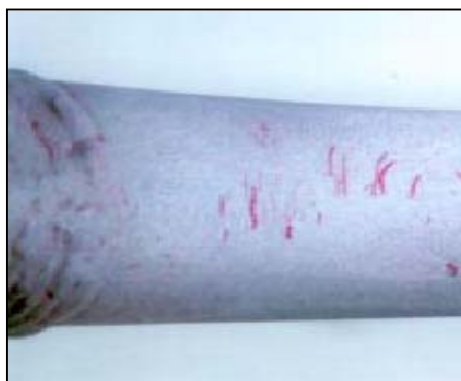
Figure 12a: Circumferential Cracking
