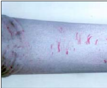
Figure A1a: Circumferential Cracking
