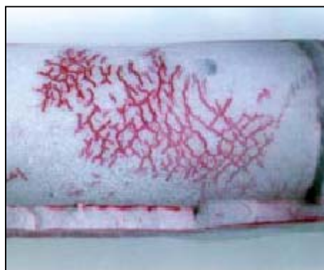
Figure 12b: Crazed Cracking
