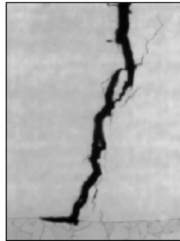
Figure A2b: Microscopic Photograph of Floor Tube Crack
