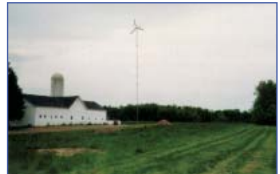
Figure 16. Bergey Excel-S/E 10 kW installed in Webster, New York.
