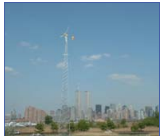
Figure 19. Bergey Excel-S/E 10 kW installed at the Liberty Science Center in Jersey City, New Jersey, with the New York skyline in the background.
