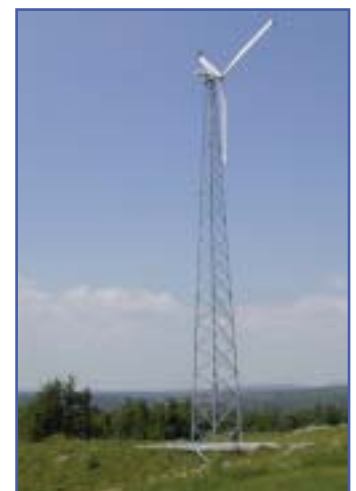
Figure 12. AOC 15/50 wind turbine at the Allen Blueberry Plant in Orland, Maine.
