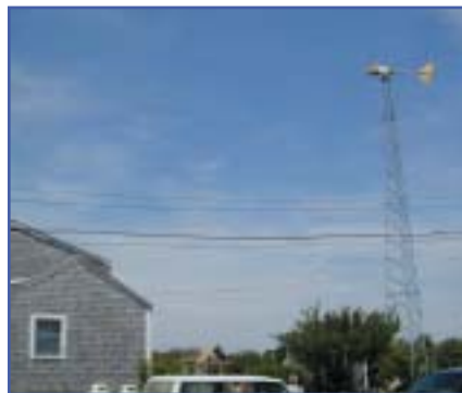
Figure 2. Bergey Excel/R 7.5 kW at the Block Island, Goose and Garden Greenhouse, Block Island, Rhode Island.
