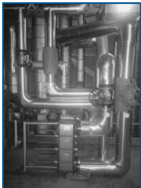
Augusta Newsprint installed a plate-style, boiler blowdown to preheat boiler make-up water.
