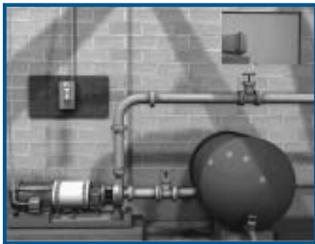
Software embedded in the controller micro-processor becomes the "brains" of a pumping system.
