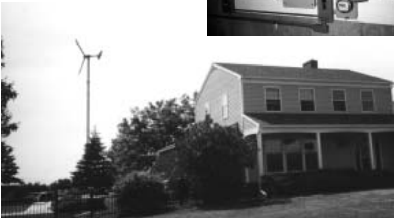
A Bergey XL.10, 10-kW wind turbine is part of a grid-connected wind/photovoltaic hybrid system that reduces the utility power used by this home in Vermont. The balance of system (upper right) includes from left to right, a Trace inverter for the PV system, a breaker box, and a Powersync inverter for the wind system.
