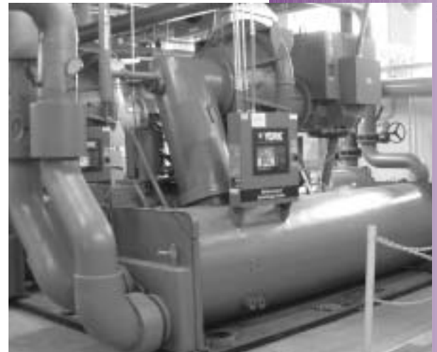
A Super ESPC helped GSA replace old R-11 chillers with new, 500-ton, R-123 chillers (one is shown here) that can serve several buildings at once at the Denver Federal Center.
