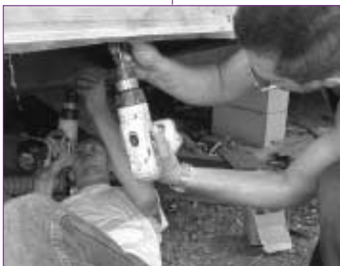
Virginia crew insulates the belly of a mobile home to increase energy efficiency.
