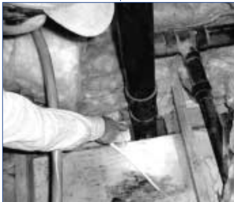
Weatherization technician encounters a common source of air infiltration.
