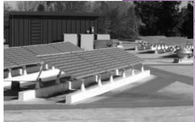
This photovoltaic energy system should provide nearly 7 kilowatts of clean solar electricity to the Sherman Indian High School campus.
