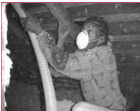
Weatherization crew blows cellulose insulation into the attic of a Nebraska home.
