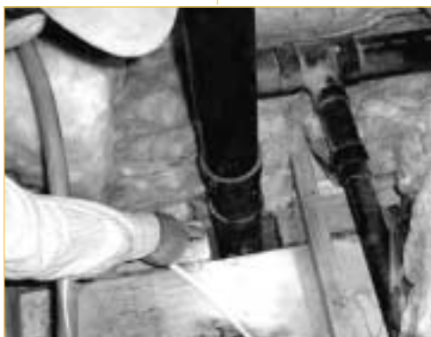
Weatherization technician encounters a common source of air infiltration.
