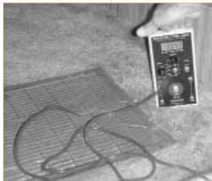
Weatherization crew diagnoses air infiltration and pressure imbalances in a mobile home.
