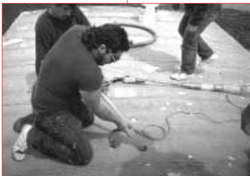
Weatherization crew blows insulation into the roof of a mobile home through a tube.
