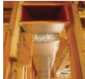
Shorter, Less Costly Ductwork
