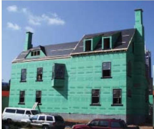
Well integrated flashing/ housewrap.
