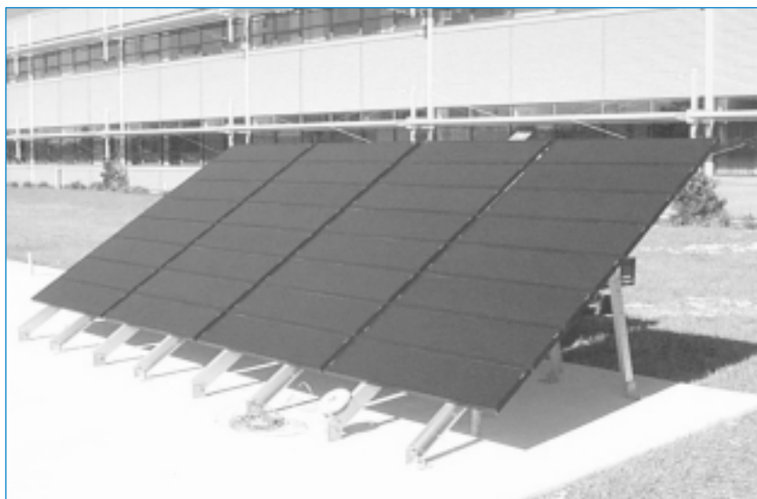
This CIS array from Siemens Solar Industries is being tested at the Florida Solar Energy Center, Cocoa, FL.
