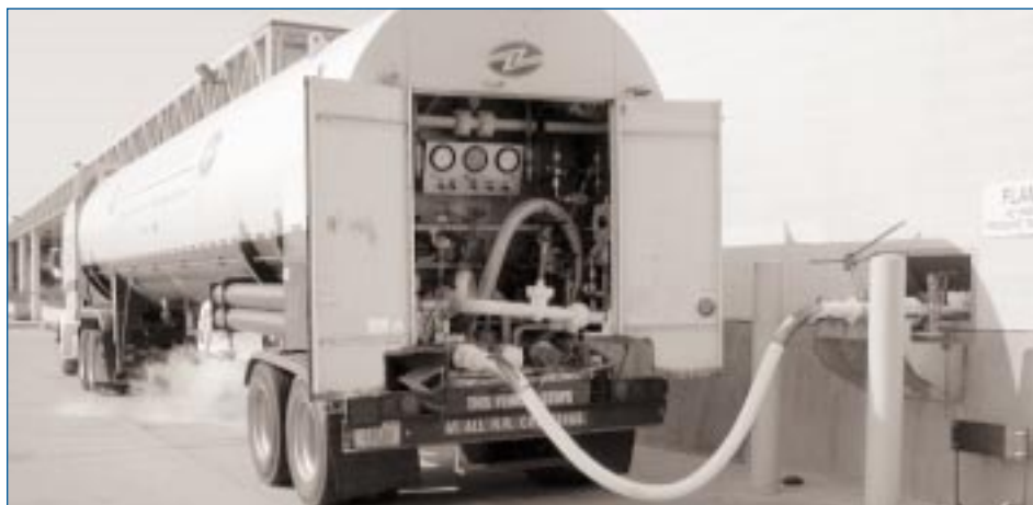
Figure 7. DART fueling station receiving bulk LNG from supply
