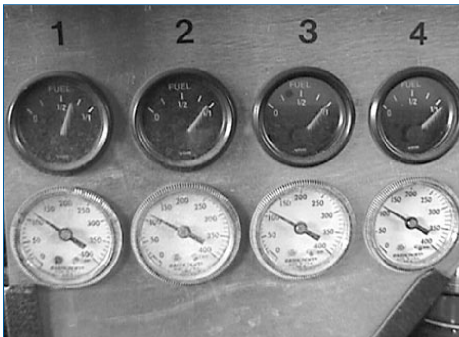
Figure 9. Fuel level and pressure indicators on LNG buses at DART
