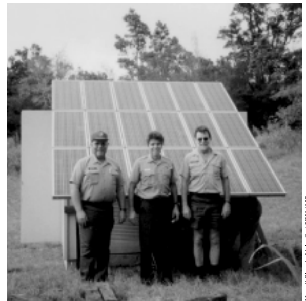
National Park Service staff in front of a modular, prefabricated portable energy shed, which includes a photovoltaic power system with an integrated propane generator, at Ainahou Ranch in Volcanoes National Park in Hawaii. This project was co-funded by DOE FEMP and Hawaii Electric Light Company, Inc.
