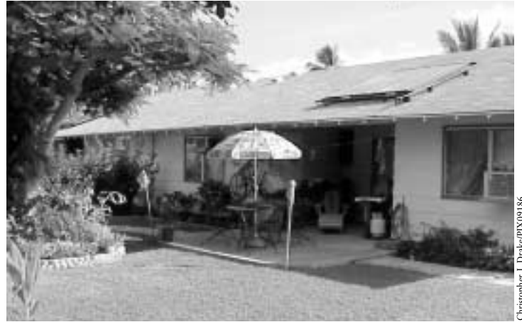
Solar water heater on military housing at Hickman AFB, Hawaii
