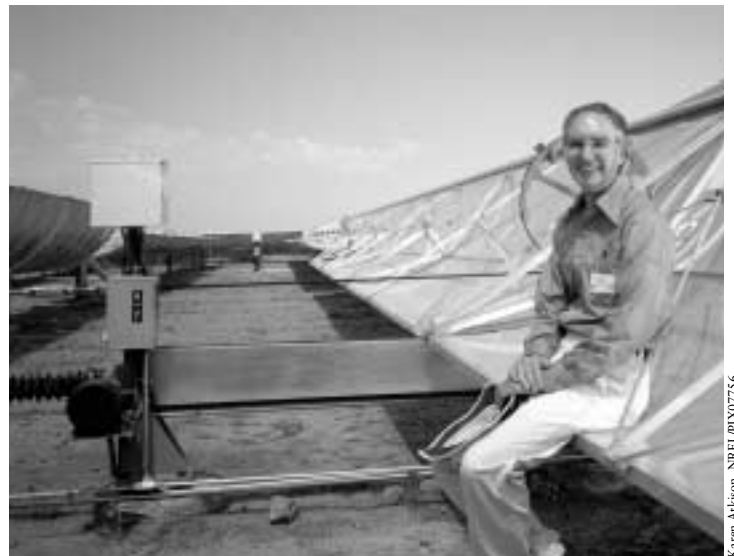
The parabolic trough water-heating system at the Federal Correctional Institute near Phoenix, Arizona
