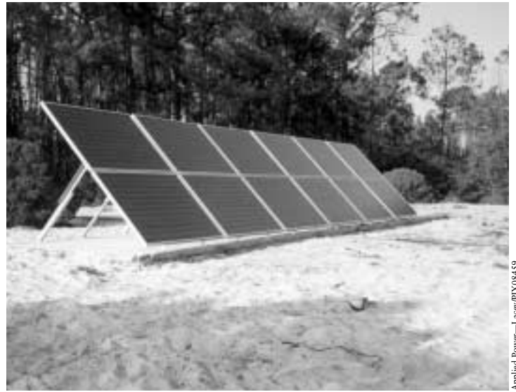
New photovoltaic system at Gulf Islands National Seashore in Florida
