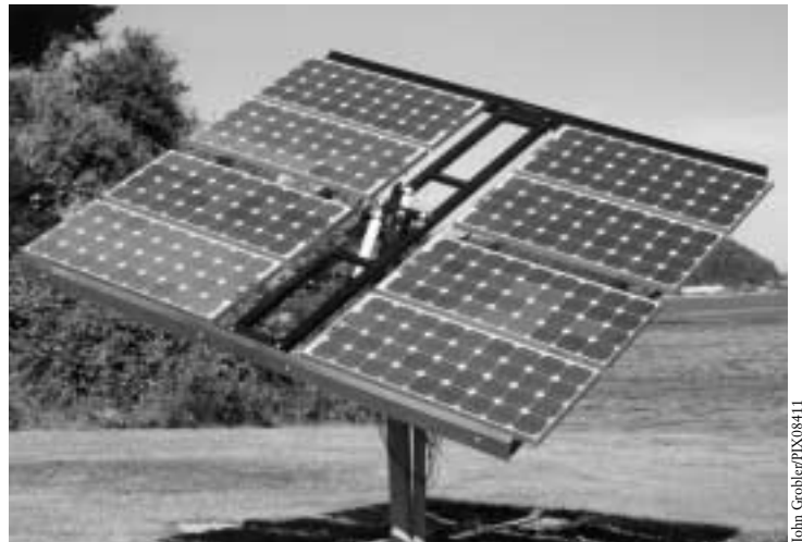
PV array installation at the EPA Region 10 Manchester Laboratory in the Pacific Northwest
