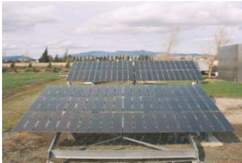
Figure 15. Retro Fitted 1.68kW Array and 2.23kW Array. (Powers STC)
