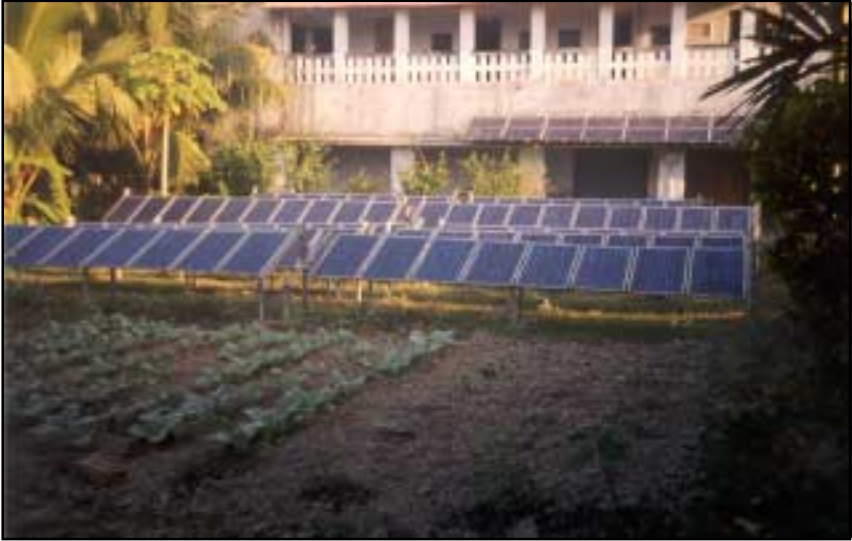
Figure 11 Battery charging station at Rupayan
