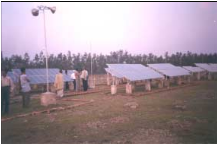
Figure 14 25kWp power plant at Sagar islands
