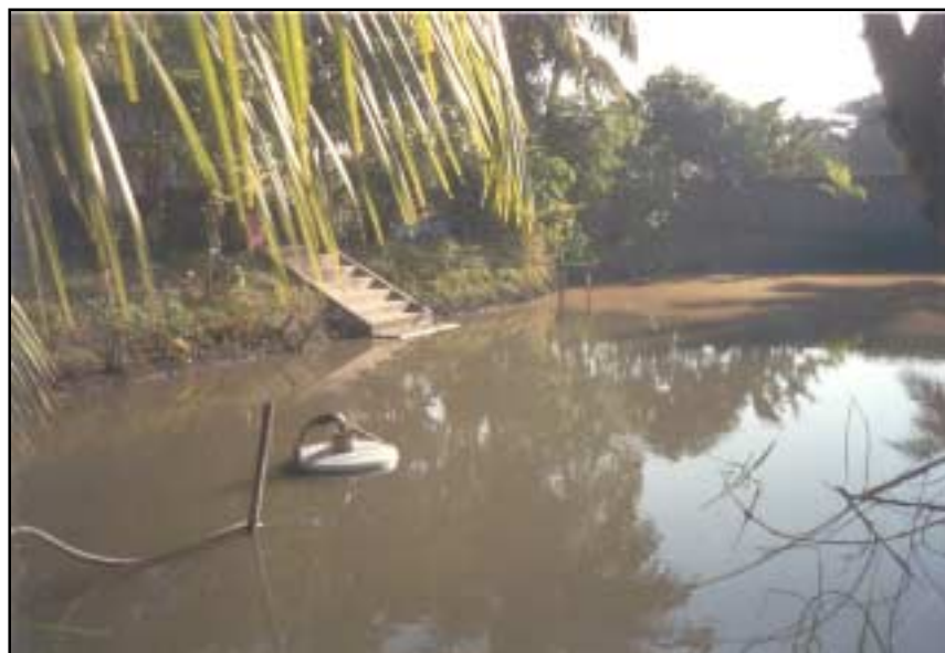
Figure 12. Water pump installed in a pond at Rupayan
