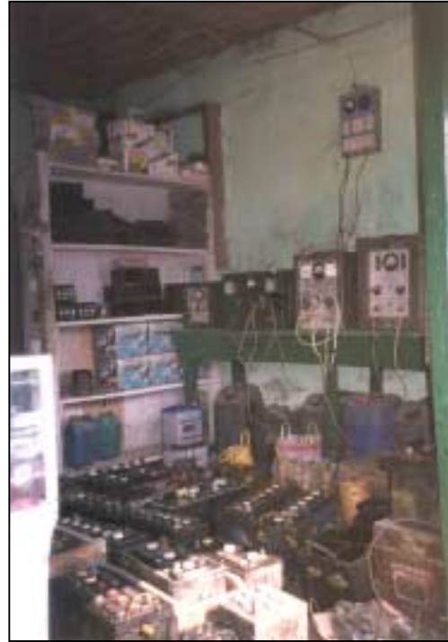
Figure 17. A typical battery charging stop using diesel generator
