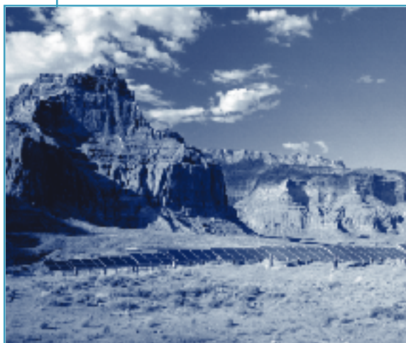
This photovoltaic test system utilizes a new generation of hybrid equipment to power Utah's Dangling Rope Marina.
