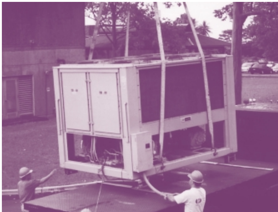
THE REBUILD HAWAII PROJECT PROVIDED FOR THE INSTALLATION OF A 400-TON VARIABLE SPEED CENTRIFUGAL CHILLER AT THE UNIVERSITY OF HAWAII.
