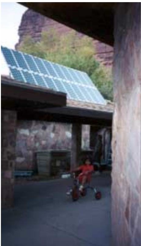
Fig. 5: This 2-kilowatt PV system was obtained recently for a school in remote Supai Village in the Grand Canyon.
